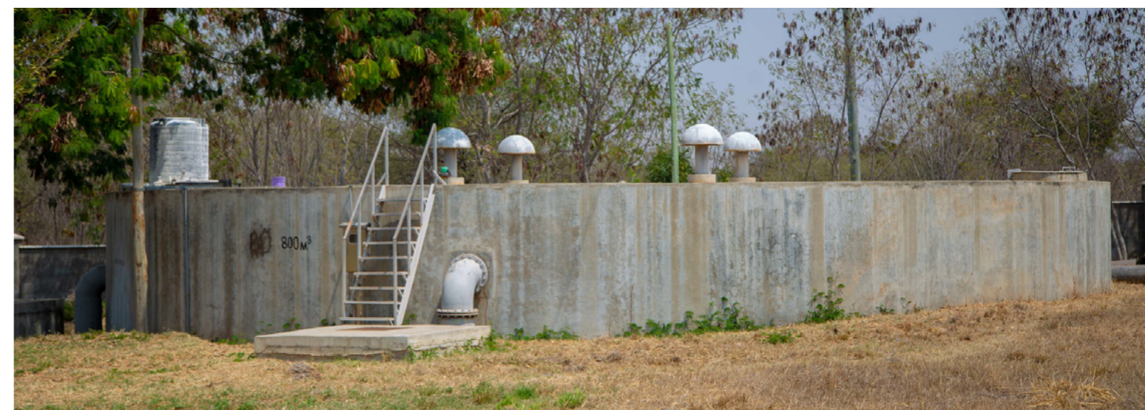
One of the water sanitation and storage facilities installed at the Mzakwe Catchment Area.
